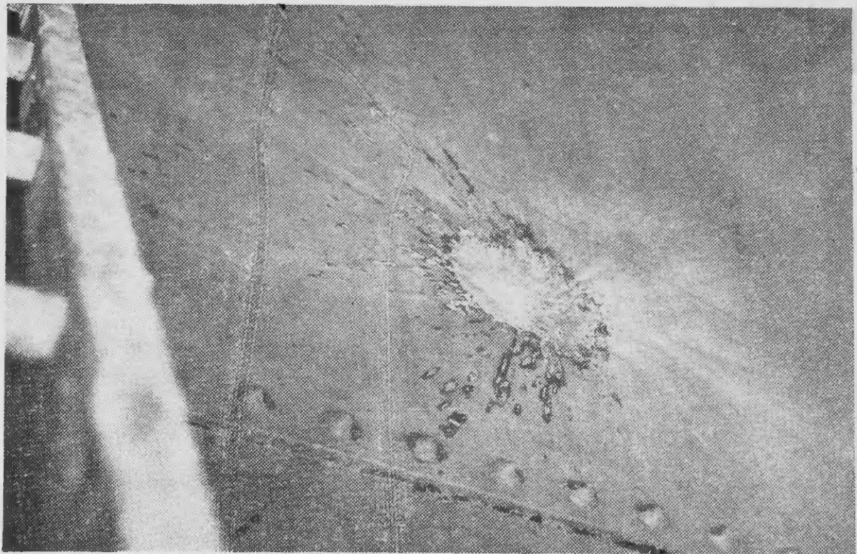
One of the first shells to strike the Western Hemisphere in World War II made this splashy dent an inch deep in tank 112 the night of February 16. Luckily it struck a glancing blow and failed to break through the tank shell. The dark line of oil leaks below the rivets shows that it loosened the seam. Officially no fragments of the shell were ever found, though early-morning souvenir hunters may have managed this.
